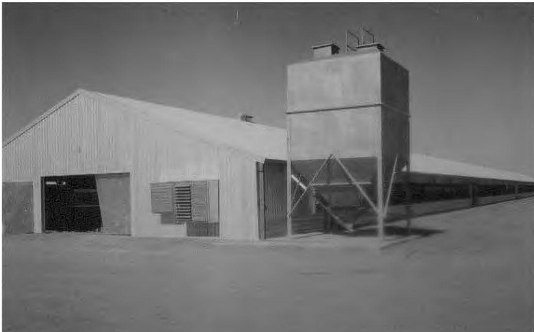
Steel Bulk Feed Tanks on Concrete Pad with Hopper Bottom
